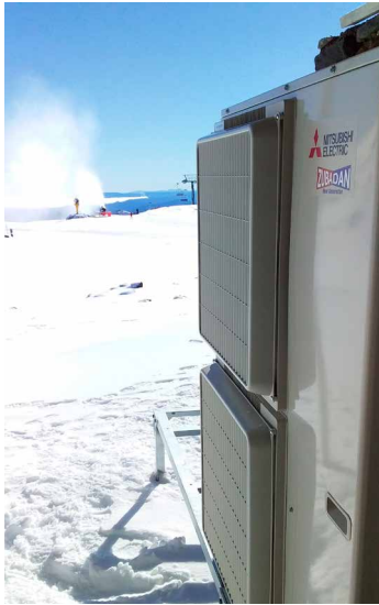
Ecodan Hot Water Heat Pump Zubadan Series installed at "The Lodge" – Ruapehu Ski Club.
